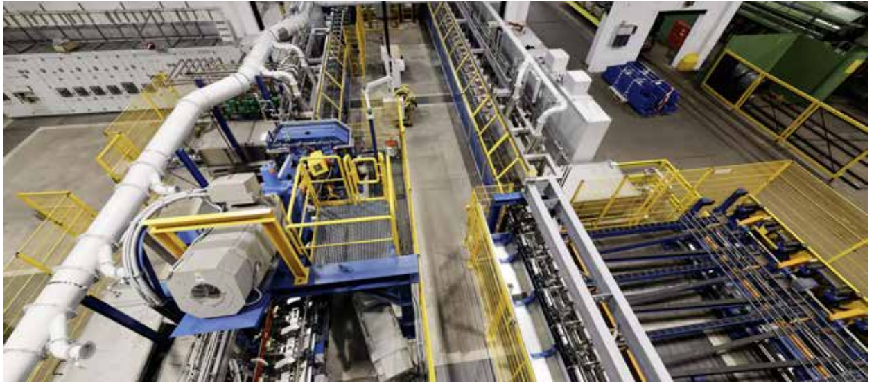
New XTP plant at Steeltec in Dusseldorf, Germany
